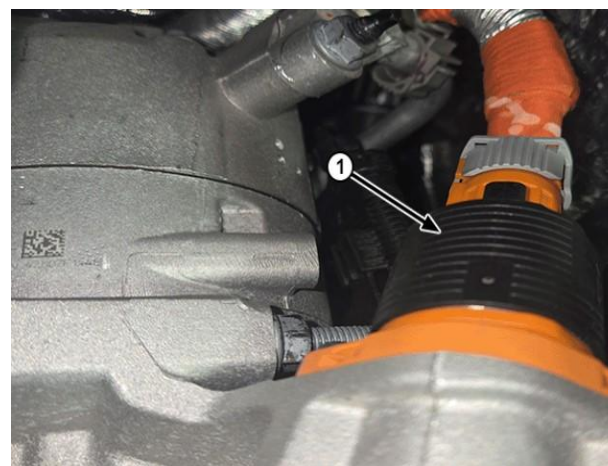
1 - A/C Compressor High Voltage Wire Harness Connector
