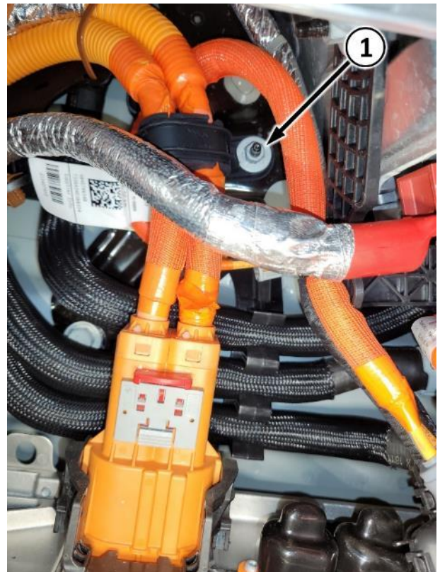
Figure 43 – HV Battery - Primary
