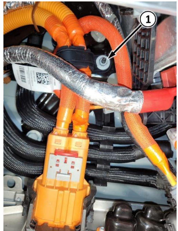
Figure 43 – HV Battery - Primary
