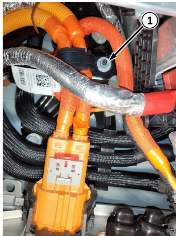
Figure 43 – HV Battery - Primary
