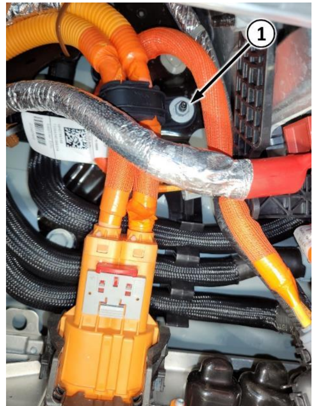
Figure 43 – HV Battery - Primary
