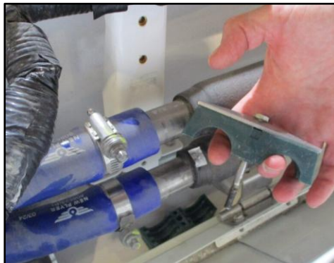
Figure 30: Twin Clamps Disconnected on Curbside of Rooftop ESS Enclosure
