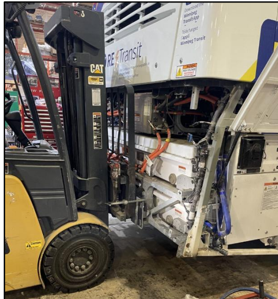
Figure 18: ESS Cradle Secured to Forklift
