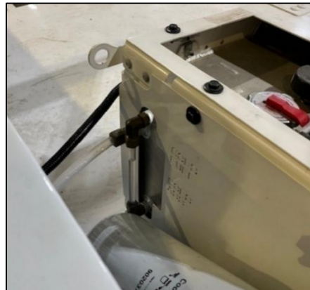
Figure 42: BTMS Sight Glass
