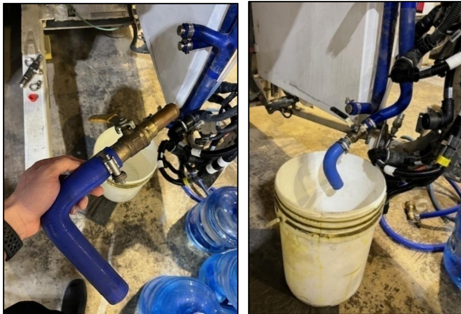
Figure 38: ESS Coolant Drain/Flush Setup
