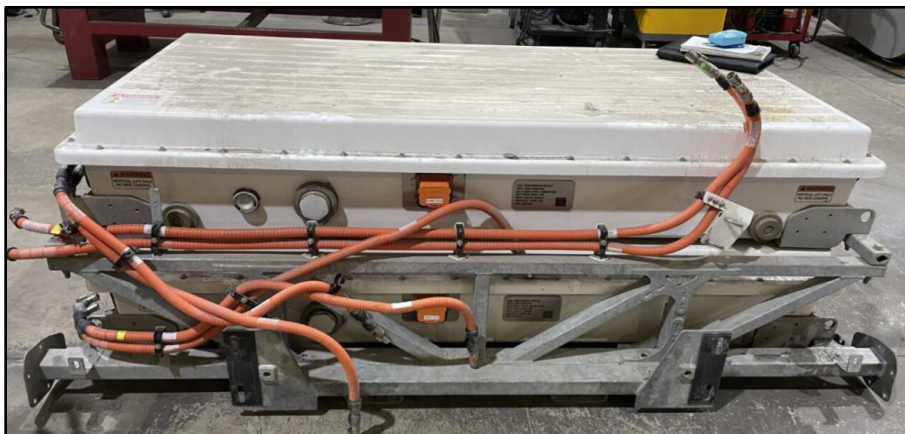
Figure 19: ESS Cradle on the Floor
