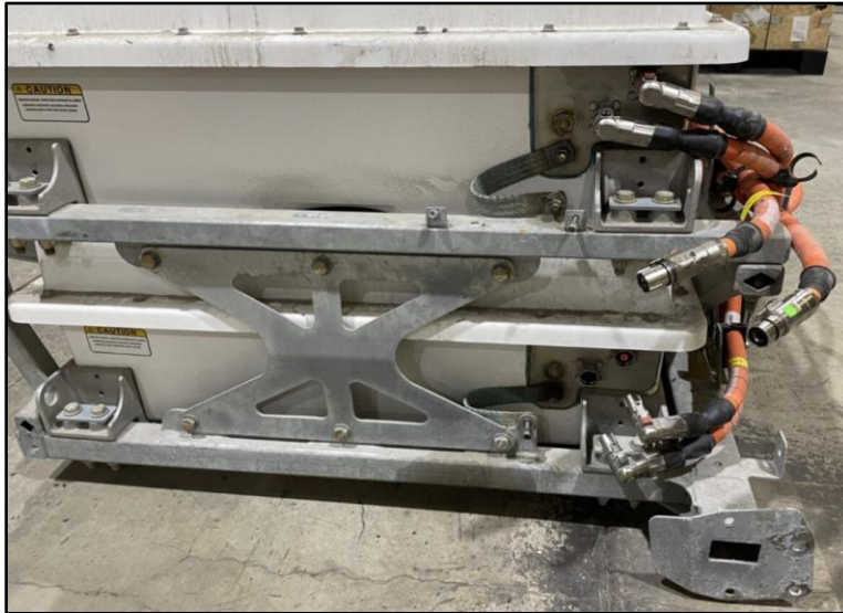
Figure 20: ESS Rack Assembly Side View
