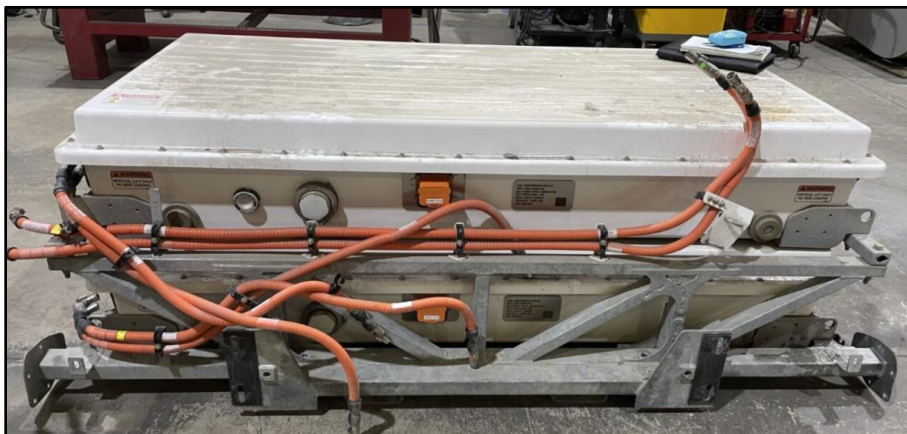
Figure 19: ESS Cradle on the Floor
