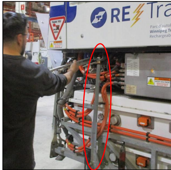
Figure 9: Loosening Strut Hardware
