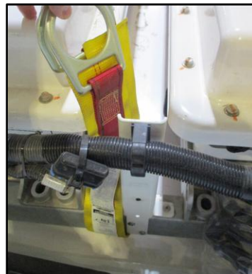
Figure 35: Safety Hook Attached to ESS Rooftop Rail
