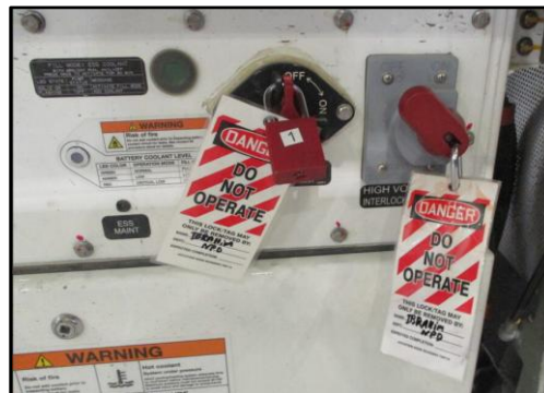
Figure 1: Main Battery & HV Disconnect Switches
