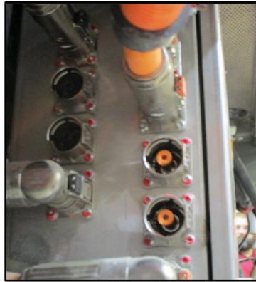
Figure 14: HV Cables Disconnected on Streetside of HV Box
