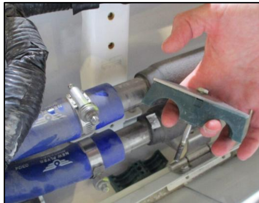
Figure 31: Twin Clamps Disconnected on Curbside of Rooftop ESS Enclosure
