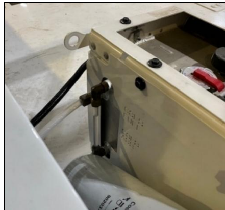
Figure 43: BTMS Sight Glass
