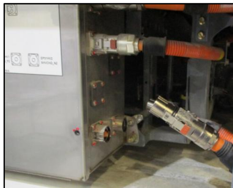
Figure 15: HV Cables Disconnected on Curbside of HV Box
