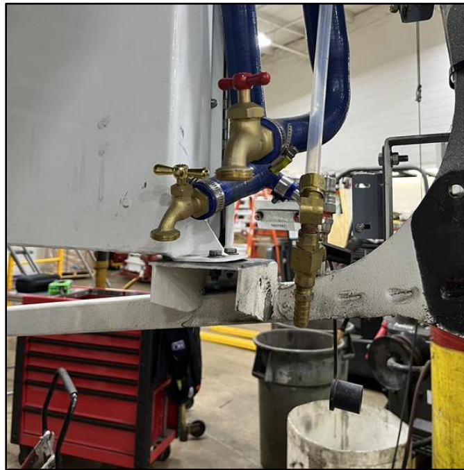
Figure 39: ESS Coolant Drain/Flush Setup
