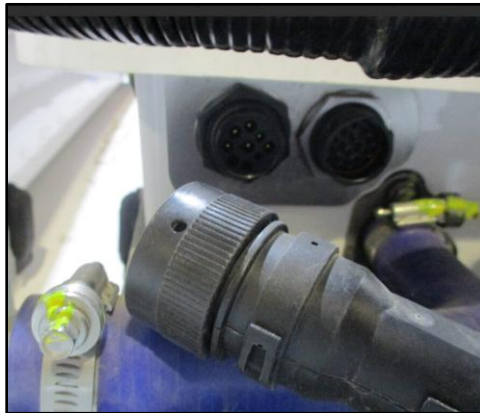
Figure 28: LV Cables Disconnected on Curbside of Rooftop ESS Enclosure
