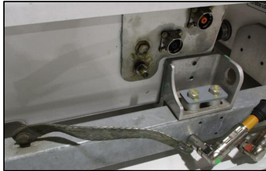
Figure 30: Ground Cable Disconnected on Streetside of Rooftop ESS Enclosure
