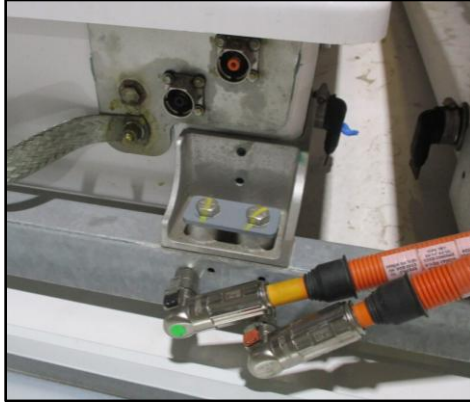
Figure 27: HV Cables Disconnected on Streetside of Rooftop ESS Enclosure
