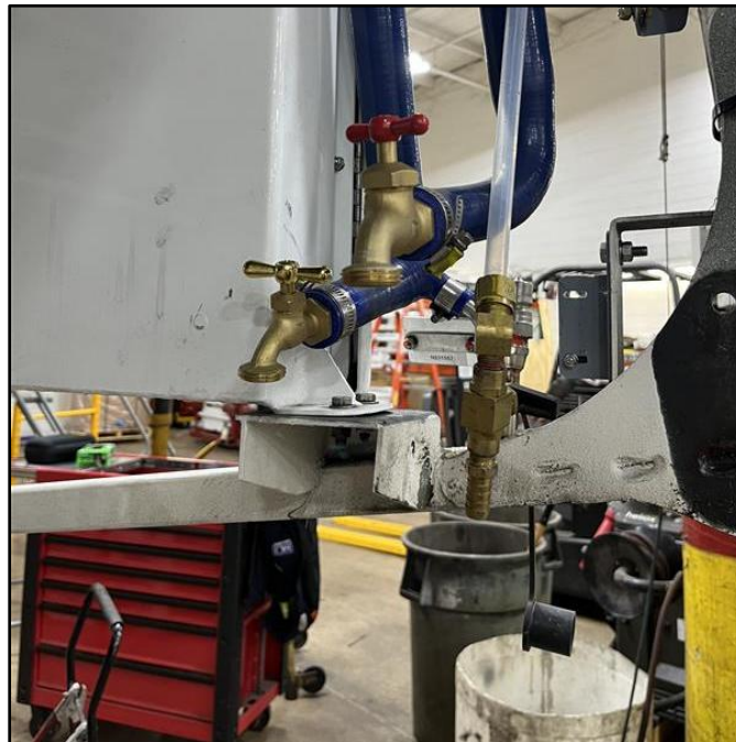
Figure 39: ESS Coolant Drain/Flush Setup
