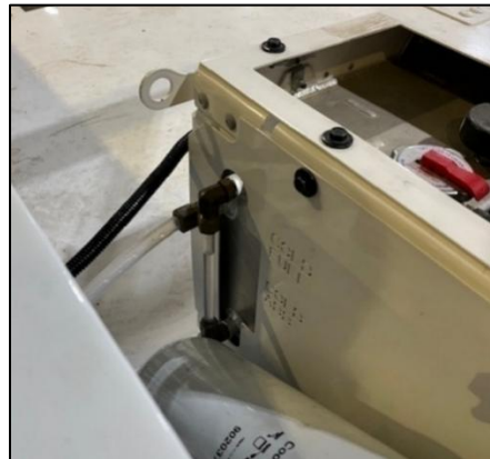
Figure 43: BTMS Sight Glass
