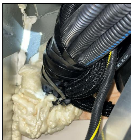
Figure 56: Jumper Harness to Rear PLC and Plywood Panel Routing
