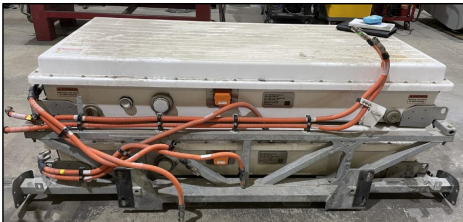
Figure 19: ESS Cradle on the Floor
