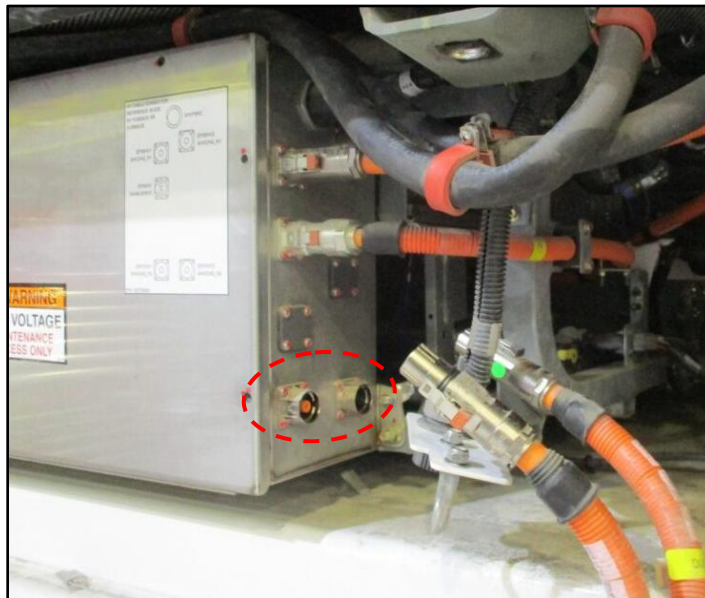
Figure 89: HV Box Curbside Connections
