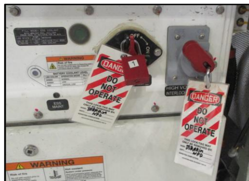
Figure 1: Main Battery & HV Disconnect Switches
