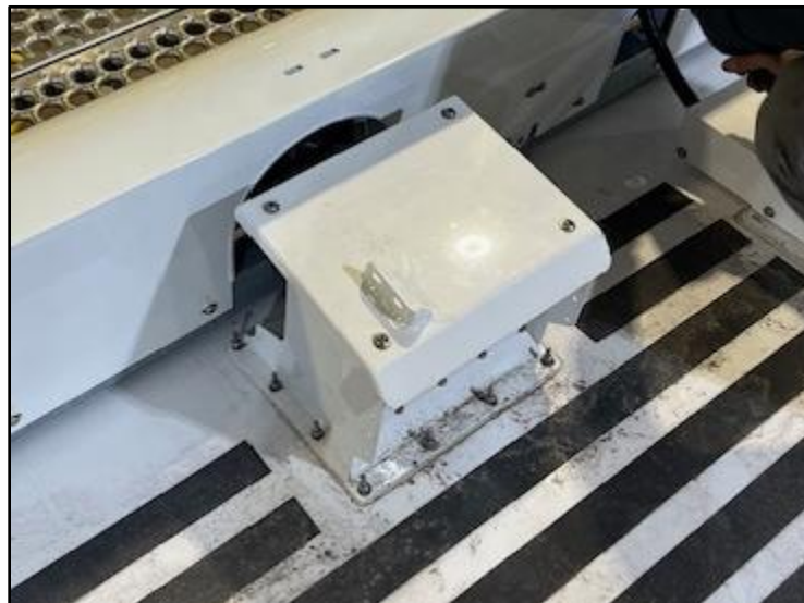
Figure 61: Reinstall Pothead Lid
