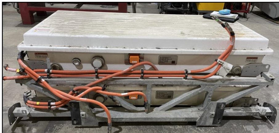
Figure 19: ESS Cradle on the Floor
