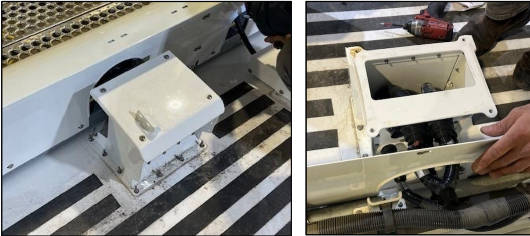
Figure 58: Rear Curbside Pothead Lid Removal
