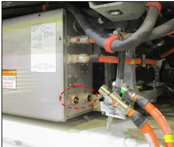
Figure 87: HV Box Curbside Connections
