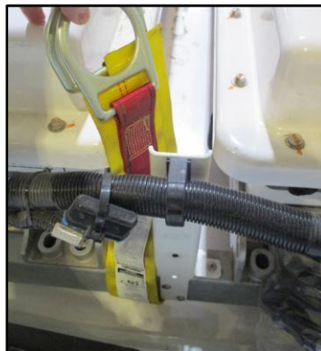
Figure 35: Safety Hook Attached to ESS Rooftop Rail
