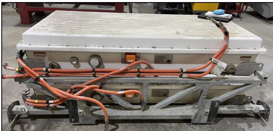
Figure 19: ESS Cradle on the Floor
