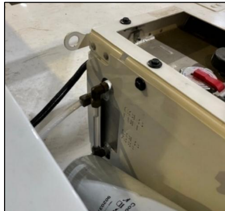
Figure 42: BTMS Sight Glass
