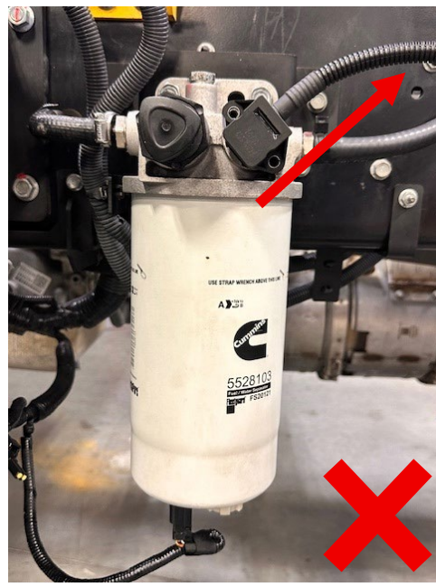
Figure 7 – Incorrectly Installed Fuel Heater
