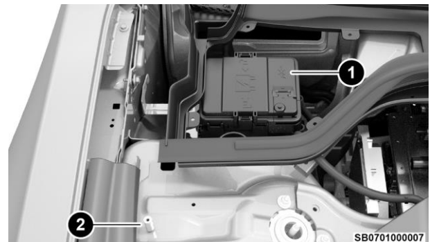
Figure 2 – Remote Battery Posts
