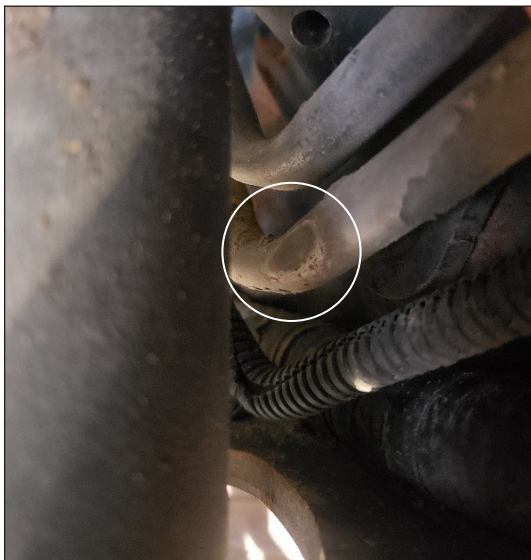
Figure 6 — Fuel Line Replacement-Level Damage Example— REPLACEMENT REQUIRED
