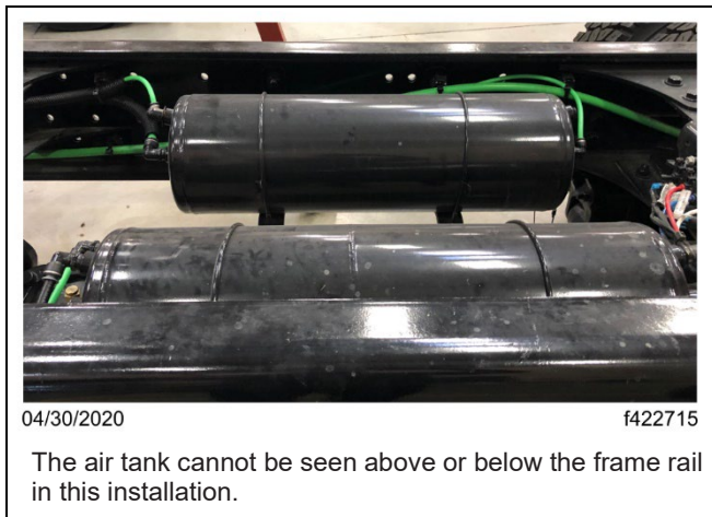
Fig. 1, In-Rail Air Tank, Top View
