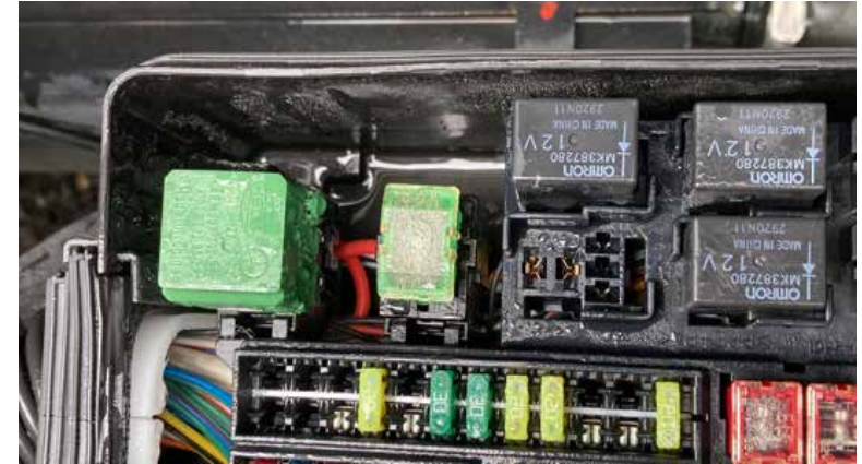
Water has reached the bottom of relay.
