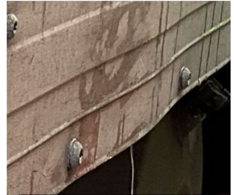
Figure 1: Baserail bulging at bottom. View from side of trailer.
