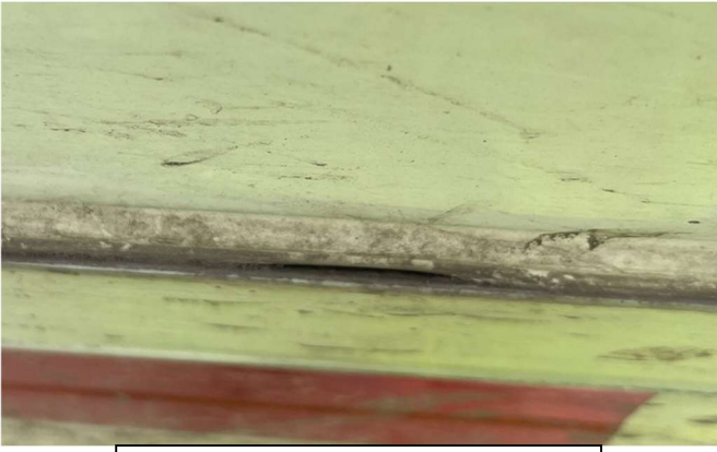
Figure 3: Caulk separation from baserail.
