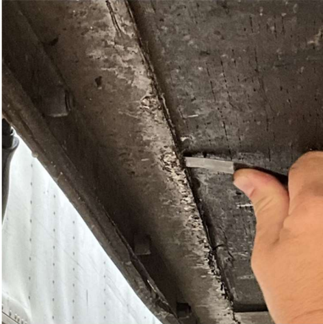
Figure 9: Floor support angle separation from floor.
