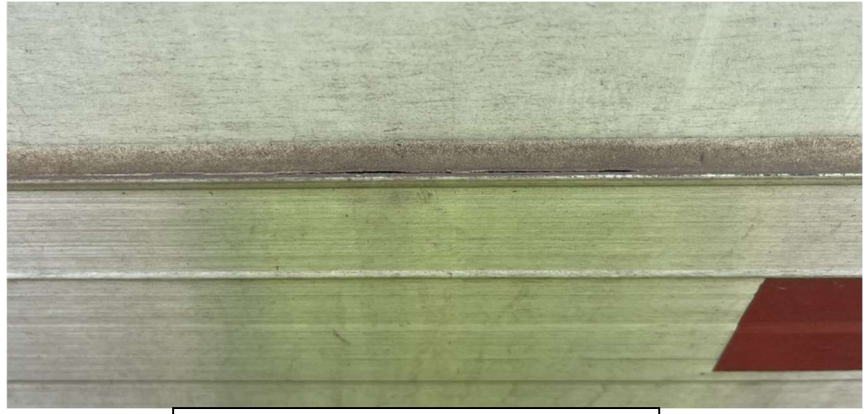
Figure 2: Caulk Separation from the baserail.
