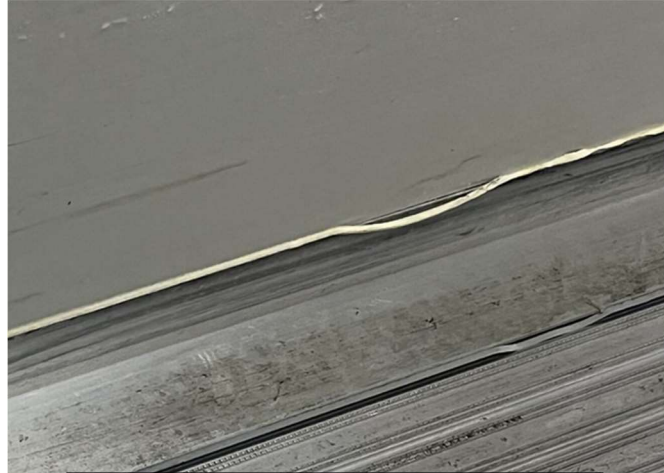
Figure 8: Interior floor angle caulk line failure.
