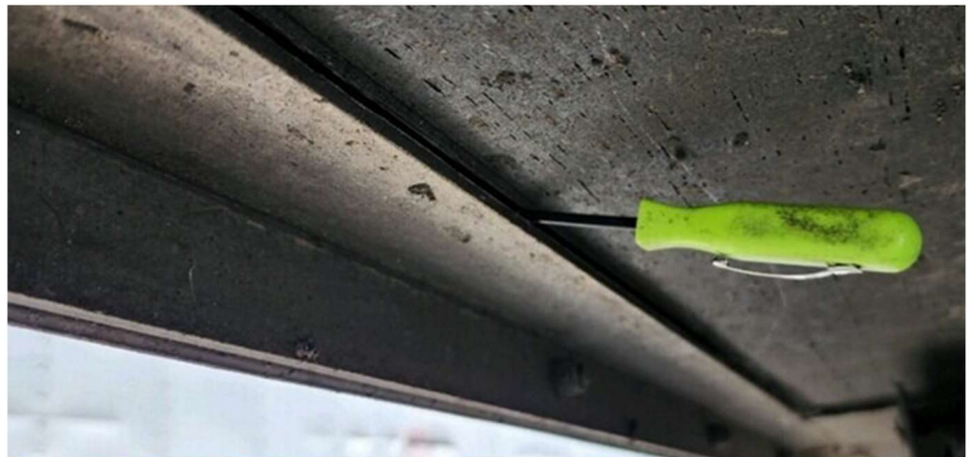
Figure 6: Floor support angle separation from floor.
