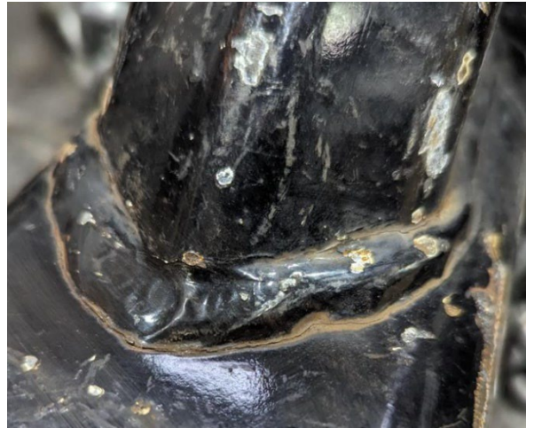
Photo 3 Example of crack near weld
