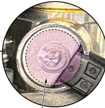
Look for leaks in this area.
