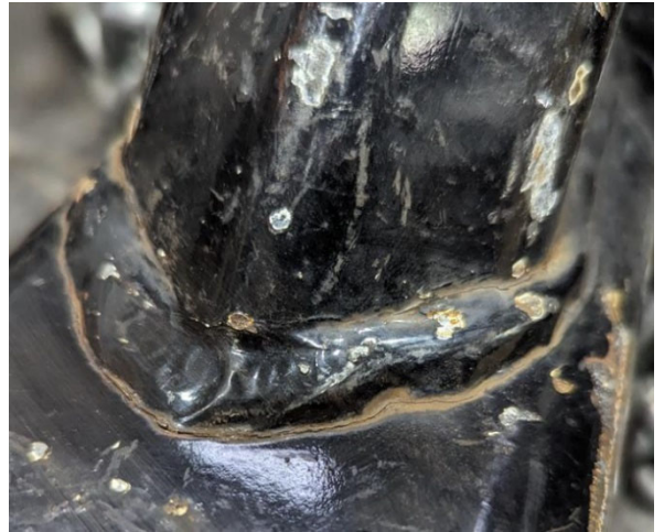
Photo 3 Example of crack near weld
