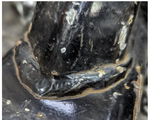
Photo 3 Example of crack near weld
