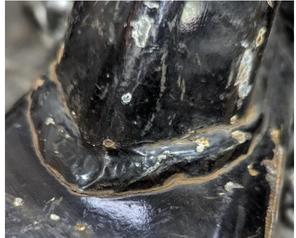
Photo 3 Example of crack near weld
