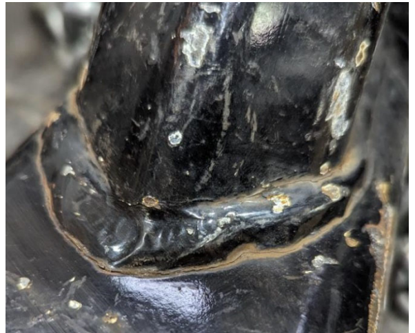
Photo 3 Example of crack near weld
