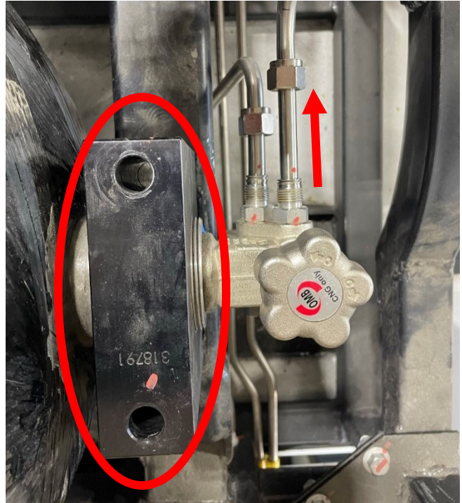
Figure 16 - Lines and bolts to be removed.
