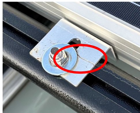
Figure 1B, recalled aluminum bracket with stress fractures & incorrect washer.
