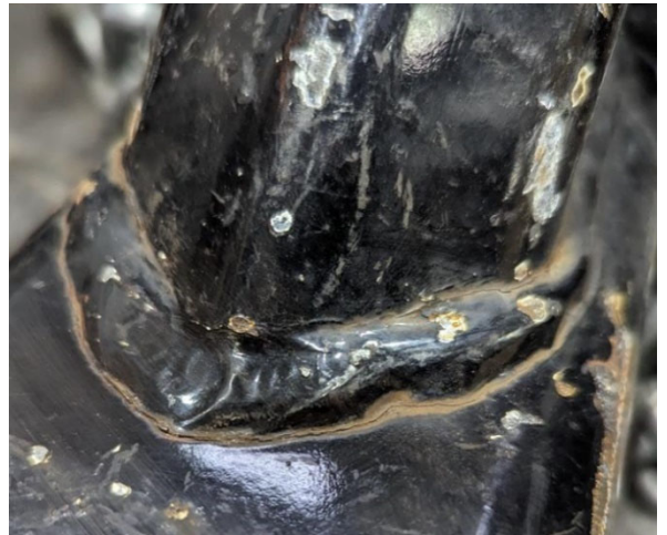
Photo 3 Example of crack near weld
