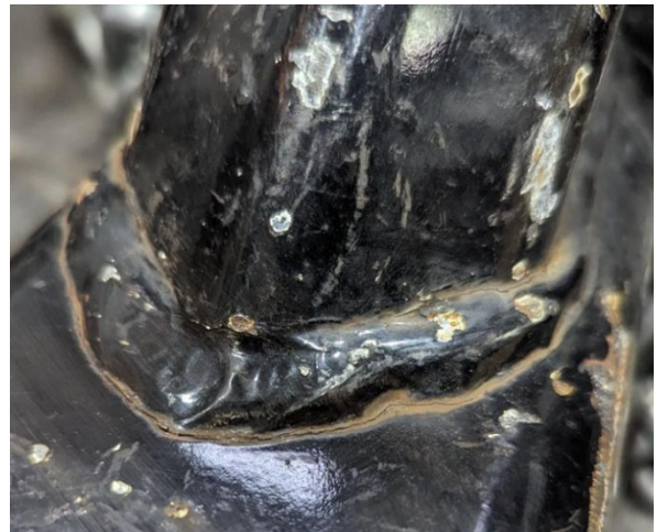
Photo 3 Example of crack near weld
