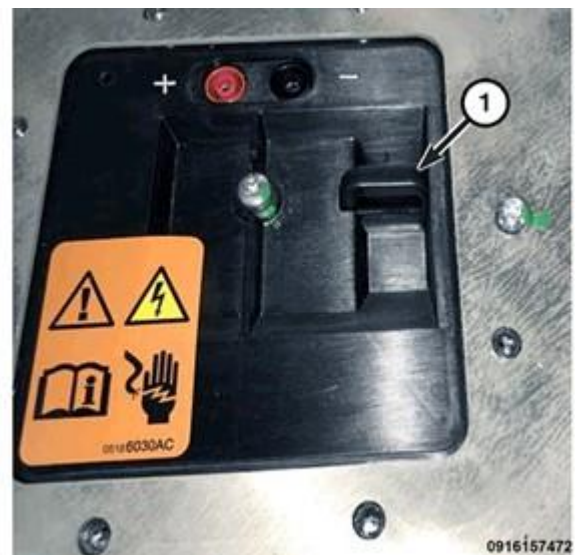
Figure 39 – Service Lockout Loop
