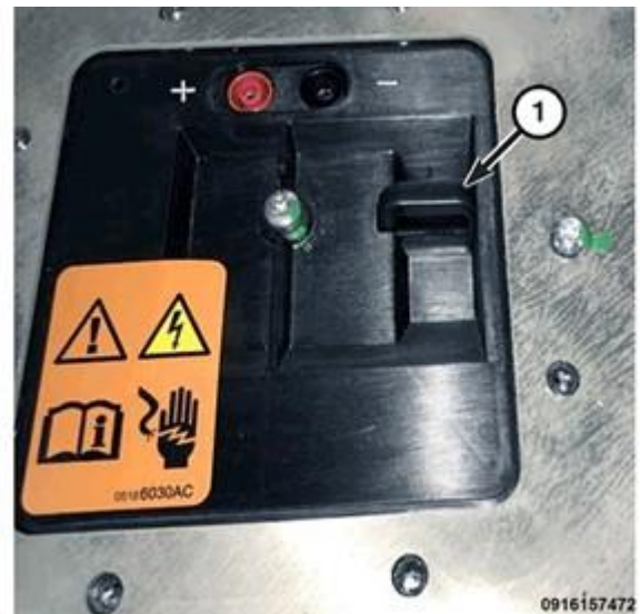
Figure 39 – Service Lockout Loop
