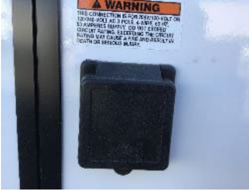
(Fig 1) 110-VOLT SHORE POWER INLET
