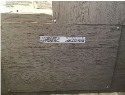
(FIG 2 – 2 OF 2) POWER INVERTER CABINET ACCESS PANEL TO POWER TRANSFER SWITCH
