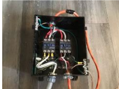
(FIG 3) 10/3 ROMEX WIRE AT TRANSFER SWITCH INCORRECT
