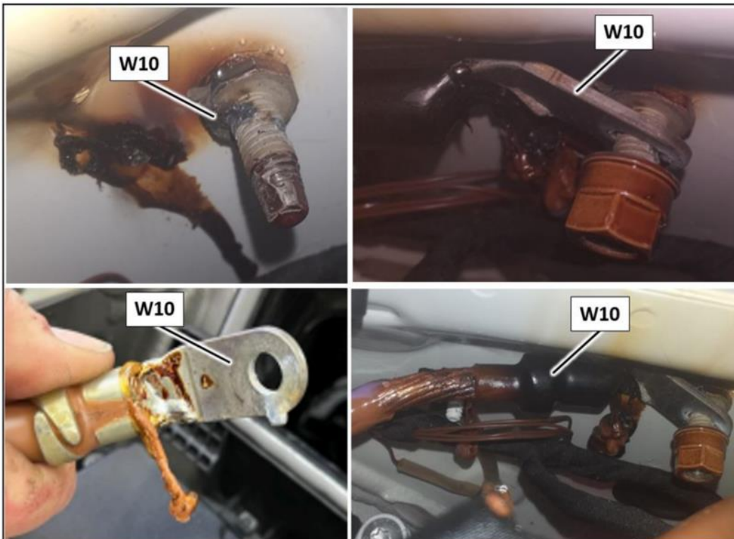
Figure 6, Example illustration of damage profiles for an on-board electrical system battery ground point (W10)
