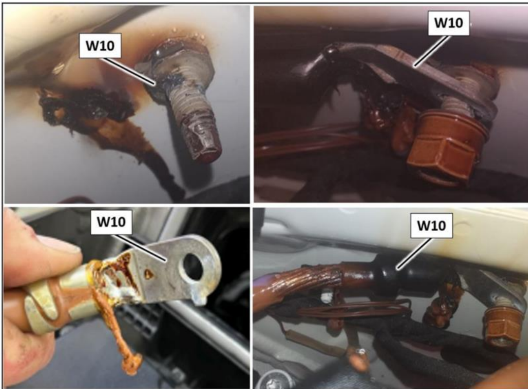
Figure 6, Example illustration of damage profiles for an on-board electrical system battery ground point (W10)
