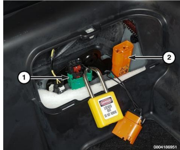
Figure 15 – Service Lockout Loop
