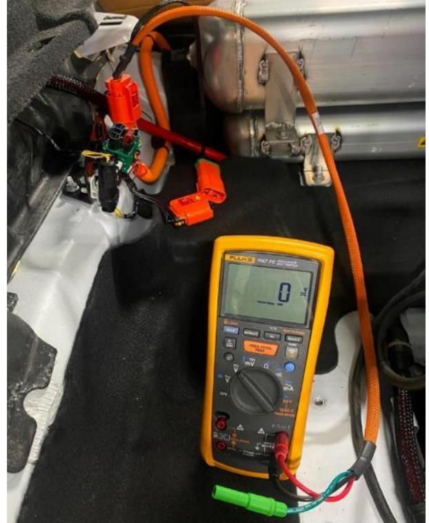
Figure 14 – PHEV Circuit Testing
