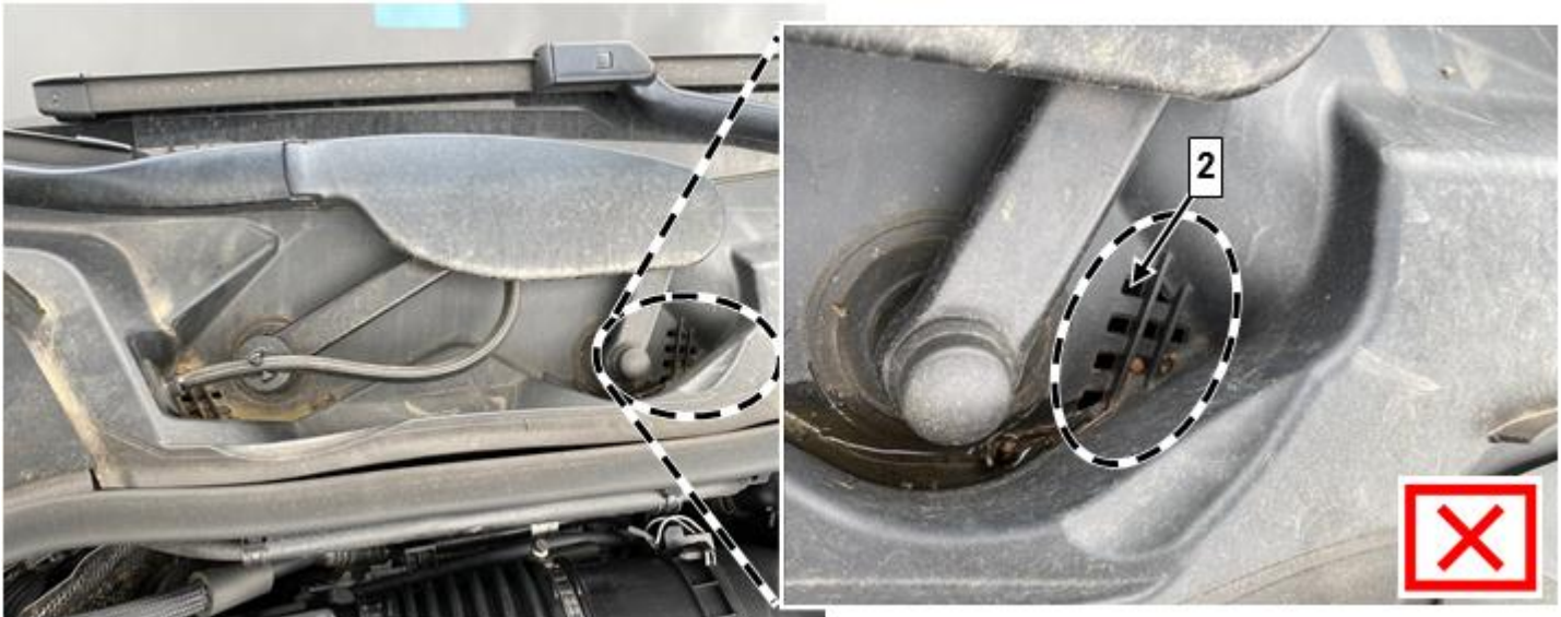
Figure 1.1 Drain of air/water duct not OK
