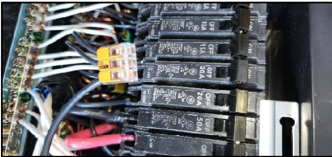
A close up of the top circle in the above photo.
