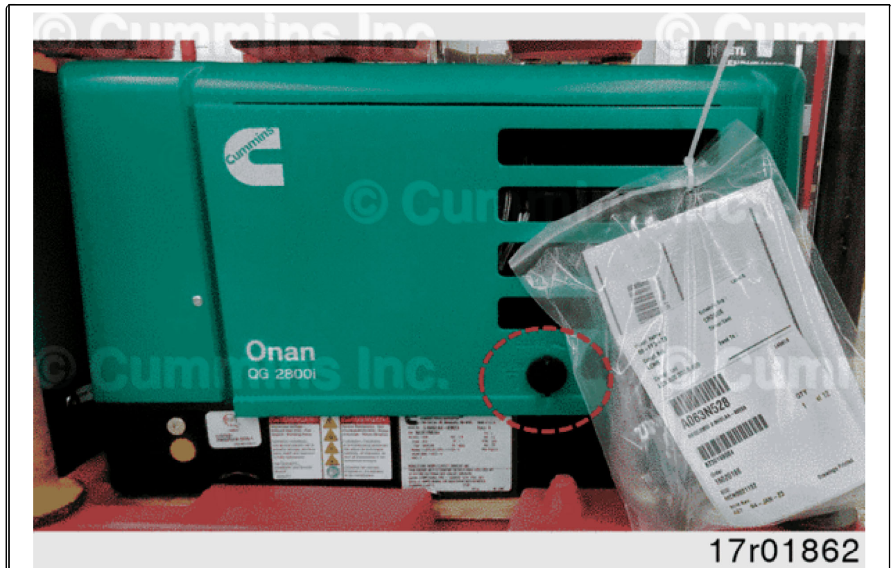
Figure 25, Generator Set After Fix
