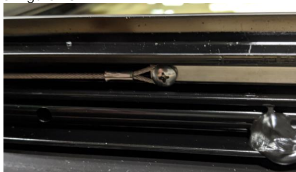
Figure 28: ER cable without slack.
