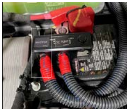
Figure 2 — Inverter Fuse Installed Under the Chassis Hood
