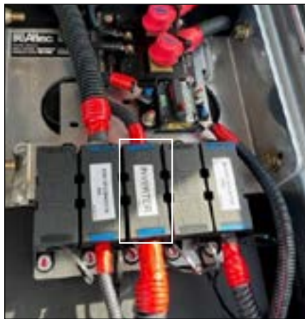
Figure 1 — Inverter Fuse Installed on Tailshelf Auxiliary Battery
