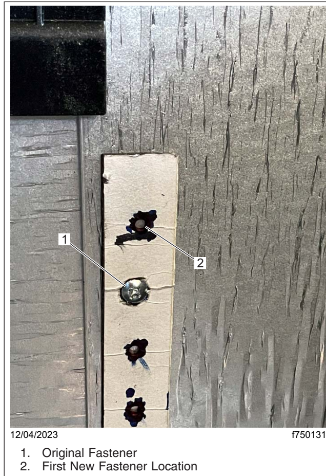
Fig. 8, Overlapped Joint Original Factory Fastener
