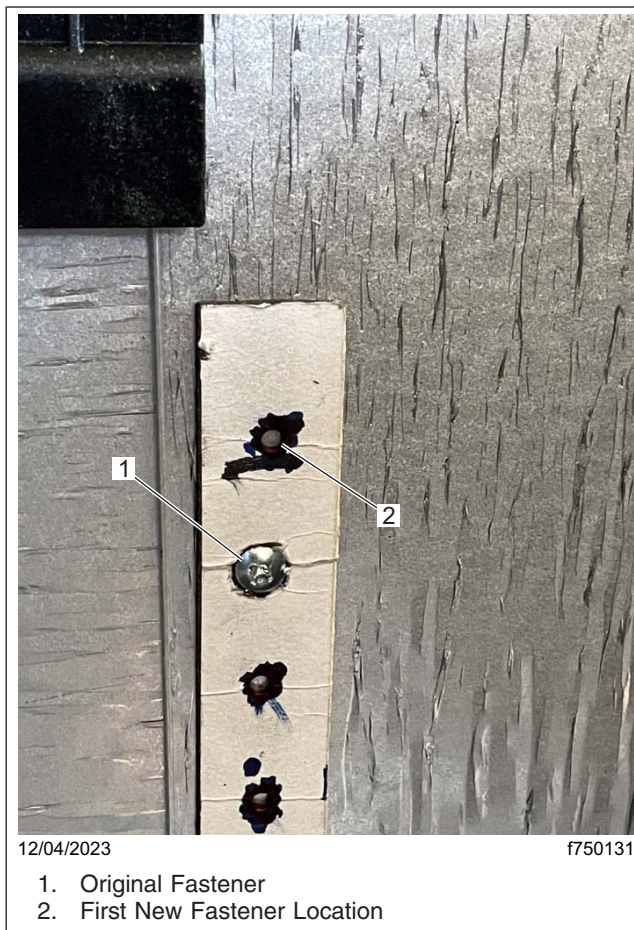
Fig. 3, Overlapped Joint Original Factory Fastener
