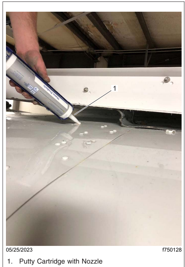
Fig. 6, Roof-Top A/C Sealed with Putty
