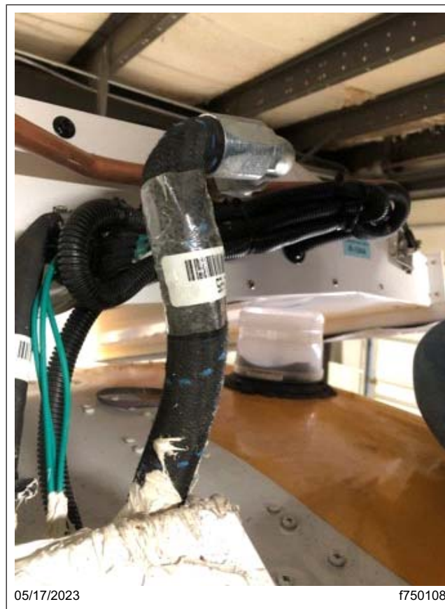
Fig. 7, Roof-Top A/C Plumbing
