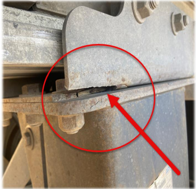
Crack on rounded edge of pan.
