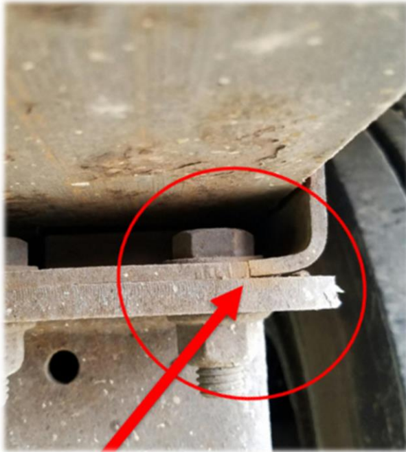
Crack near the inside bolt.
