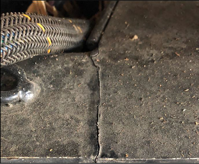
Example: Vertical surface crack – contained within template (refer to template on next page)
