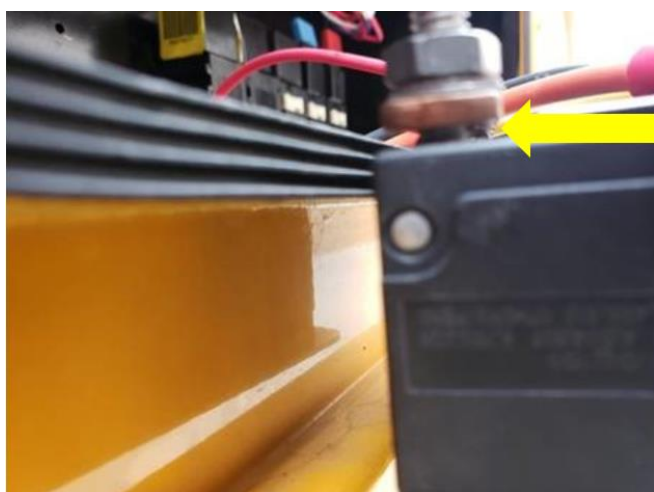
(Photo B) Incorrect
