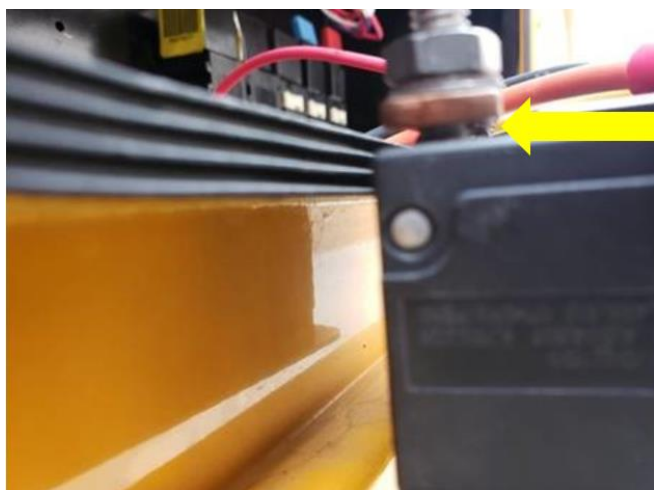
(Photo B) Incorrect
