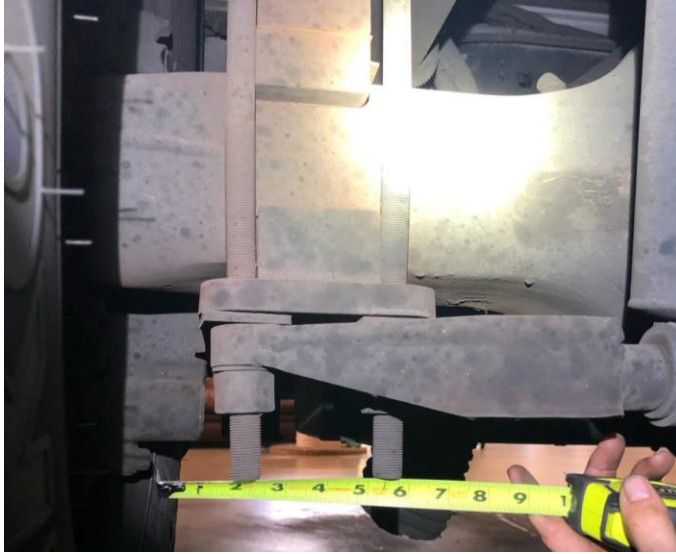
Figure 2: Bracket shown has incorrect spacing. Note U bolts not parallel.
