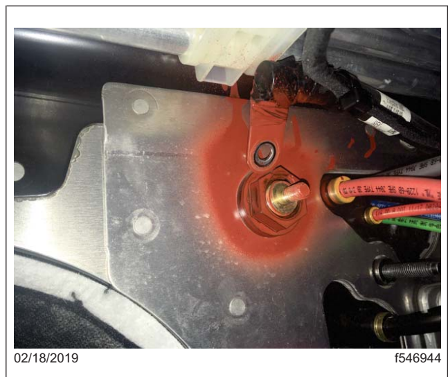
Fig. 7, GNDE Engine-Side Pass-Through Stud
