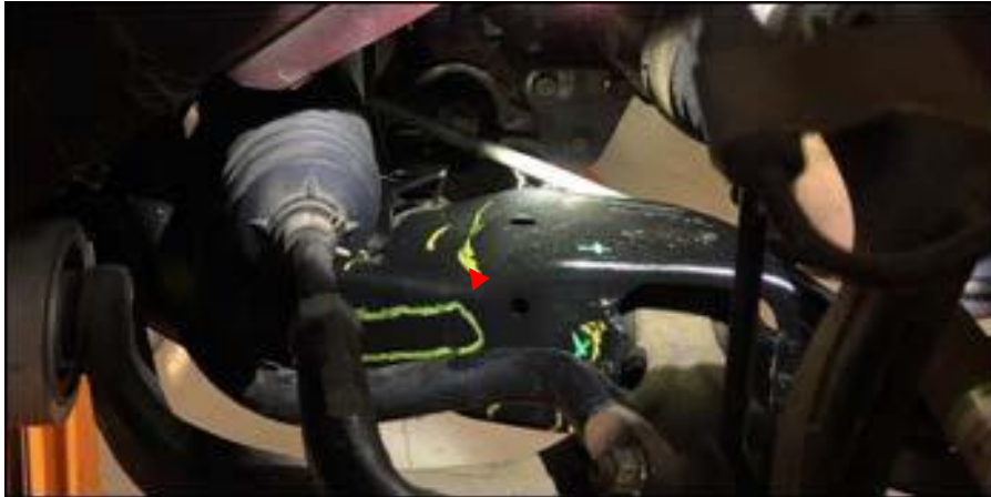
Top Side View: Non-Damaged Cross Member
