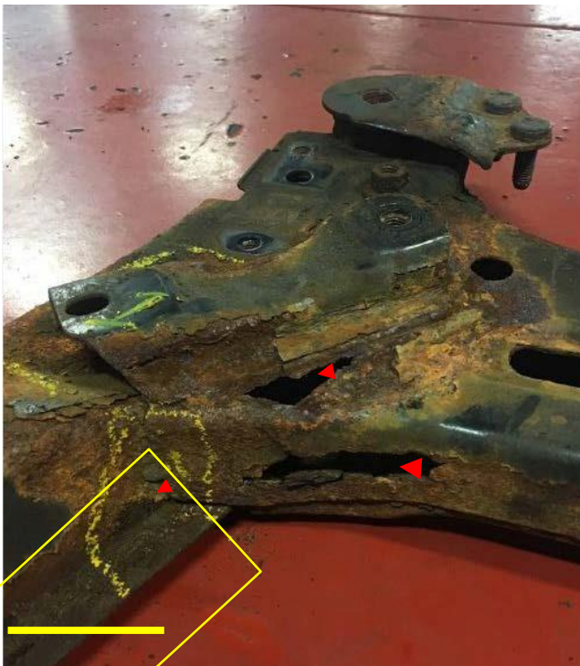
Inside Top View: Damaged Cross member
