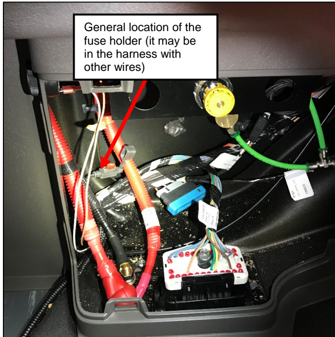
Figure 2: In-Line Fuse Holder Location
