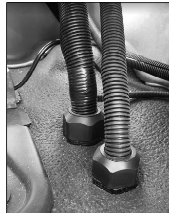
Figure 5 — Wire Going Through Wall
