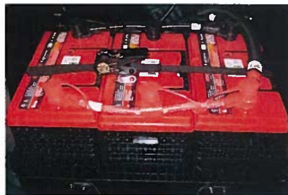
THREE ODYSSEY BATTERIES
